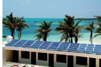
5,6 kW PV array of a PV-Wind-Diesel hybrid system installed at the Biodiversity Reserve on Contoy Island, near Cancun. [PHOTO: CONERGY MEXICO]
